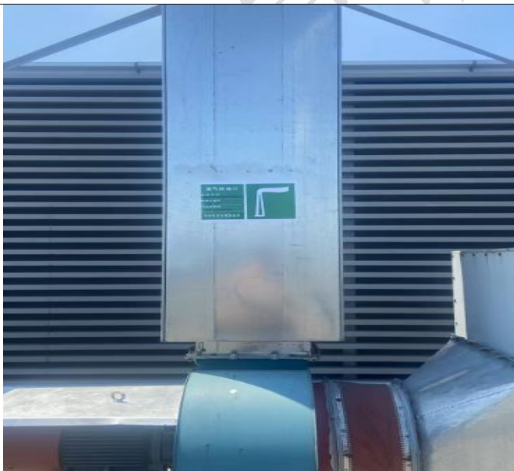
废气排放口标识标牌
